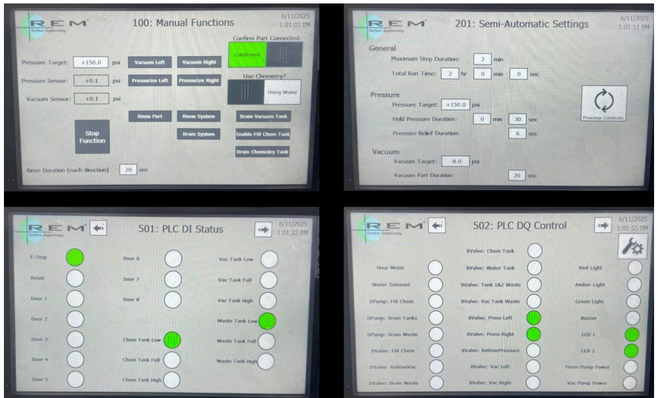
Figure 6: REM's auto declogger system with automatic control panel.
